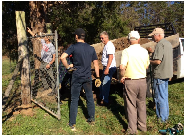
As you can see we had a great deal of good help, Herman Almond also had the right equipment for the job. A dump truck brought in a load of dirt.
